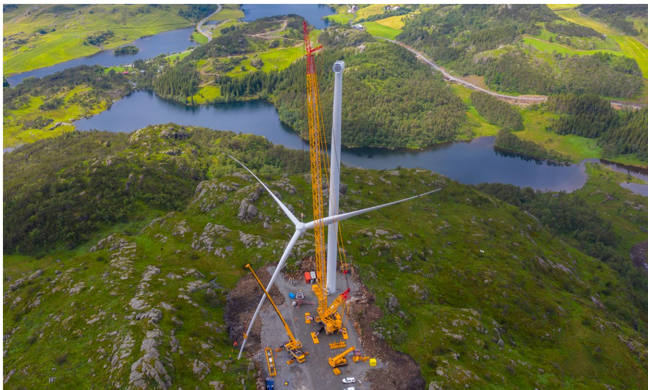
Eolus does not do any contracting work. The company's role is to manage the construction, and serve as client for the project's contracting, electrical grid and turbine or solar panel suppliers. The Stigafjellet wind farm in Norway.
